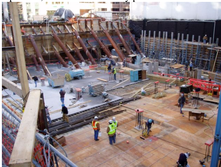
Figure 1 – Parking Garage During Formwork/Reinforcing (Notice the Rakers along the west wall in the upper left of the photo)
